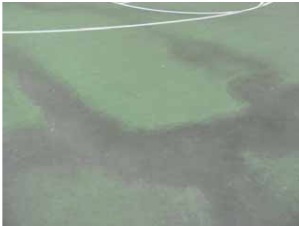
Basketball court – Note discoloration
