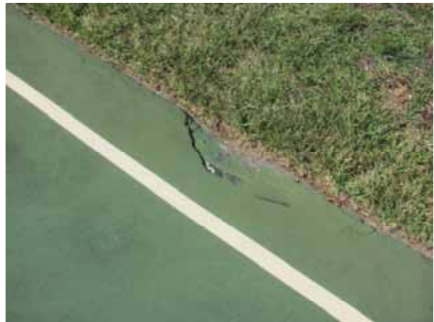
Basketball court – Note edge crack
