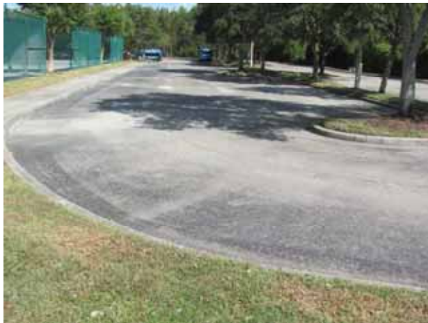
Asphalt pavement at clubhouse – Note faded seal coat
