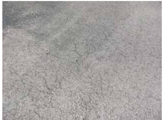
Asphalt pavement at clubhouse – Note cracks
