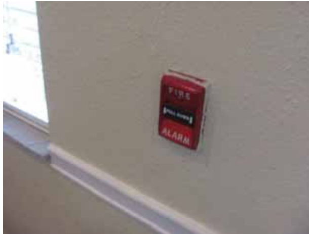
Life safety system emergency device
